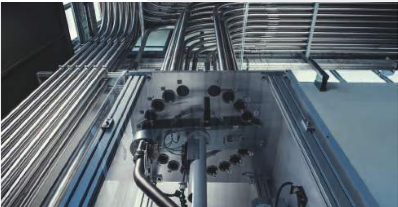
PP branching under presses.
